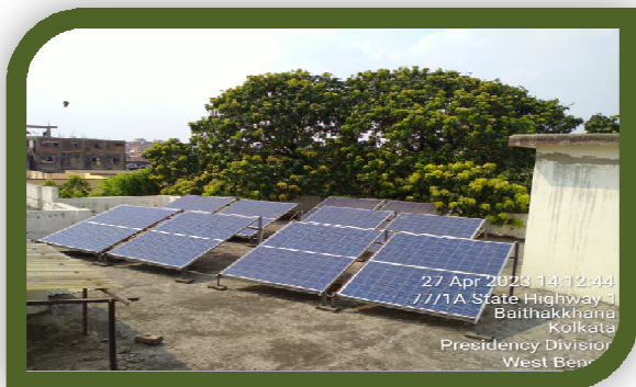
Solar panel on the rooftop Of A.J.C. Bhawan (Science Building)
