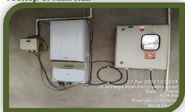
Grid connections on the rooftop of K.M. Hall
