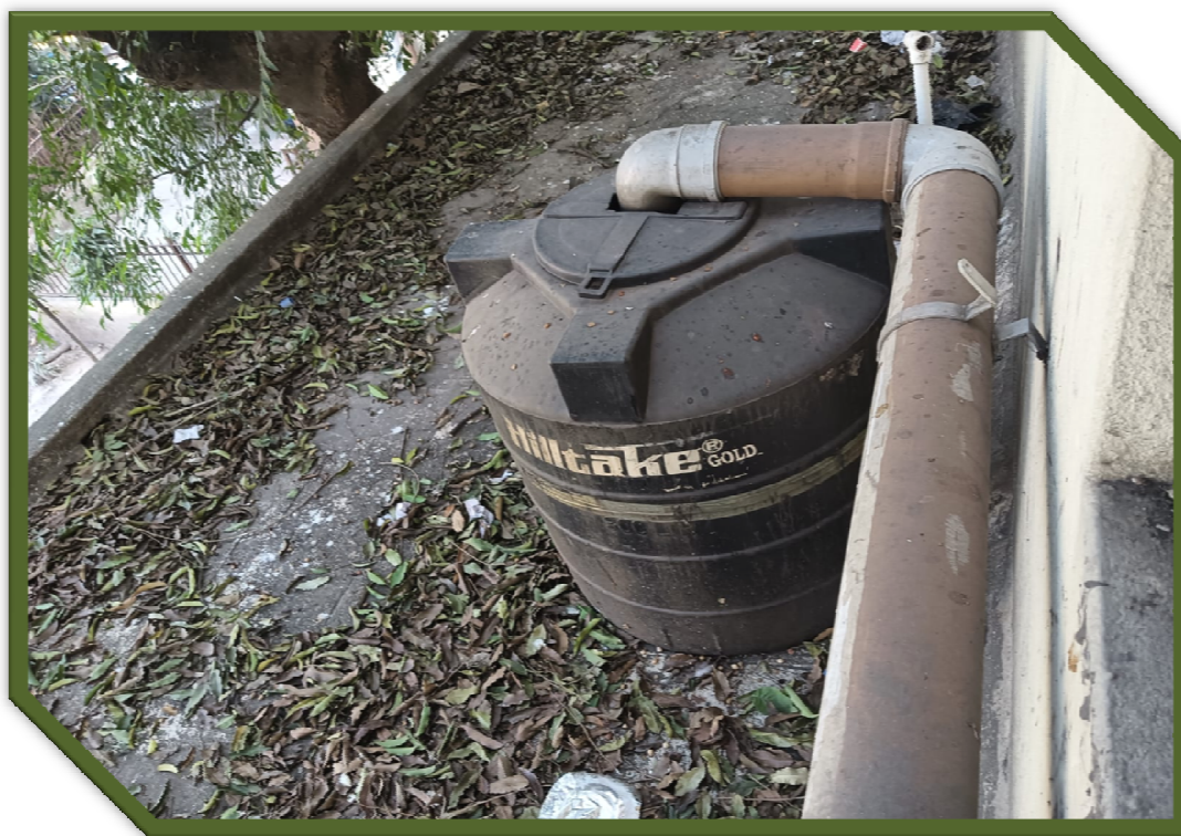
Fig. 8 : Rain water Harvesting Tank
