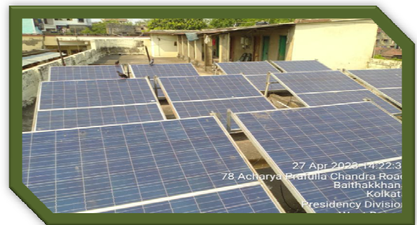
Solar panel on the rooftop of K.M. Hall
