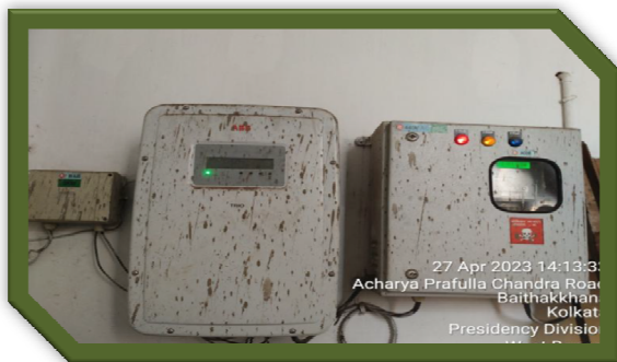
Grid Connections on the rooftop Of A.J.C. Bhawan (Science Building)
